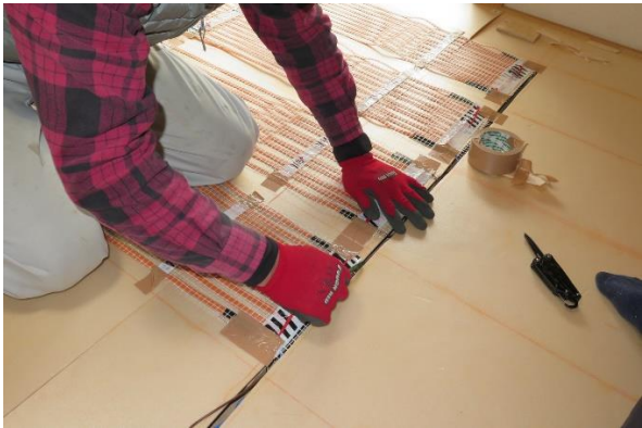
Electric Cable Routing
